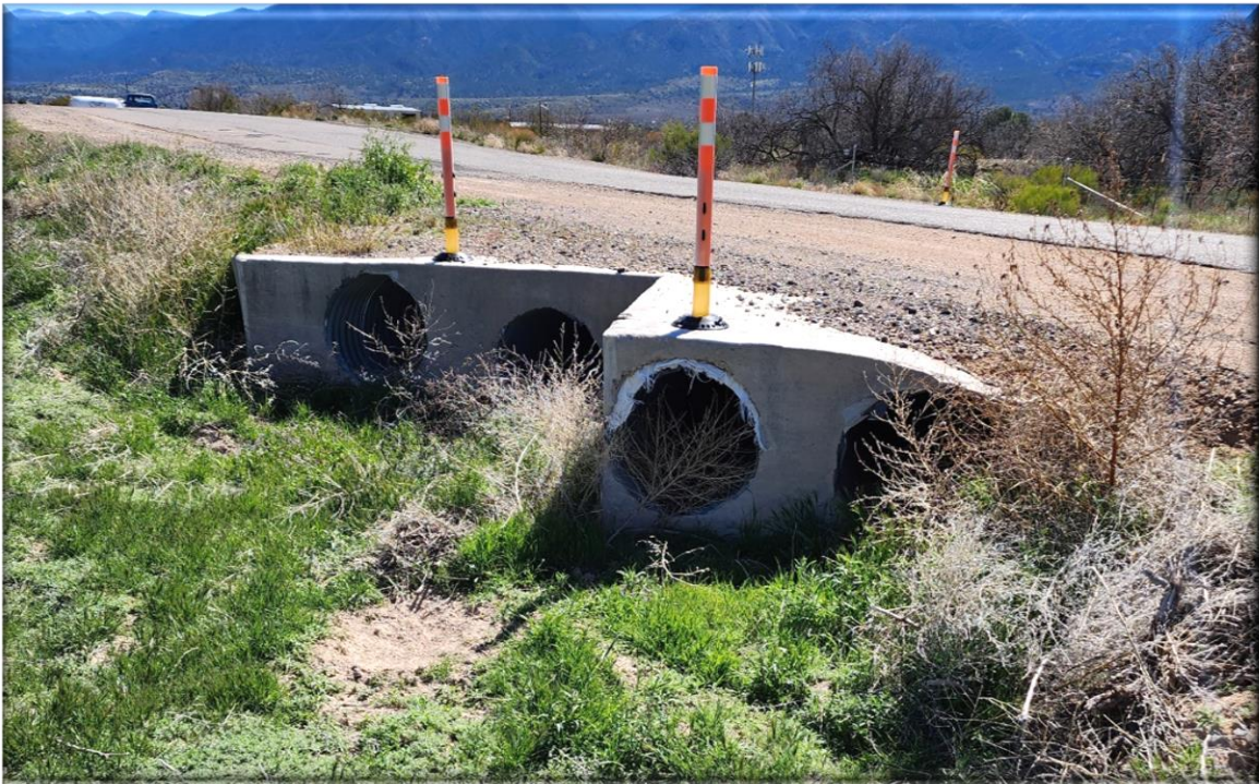
The town engineer advises that these culverts need to be upsized to accommodate necessary outflows of the retention basin to prevent stormwater overtopping the asphalt at Cowboy Trail. See bottom photo, next page.
