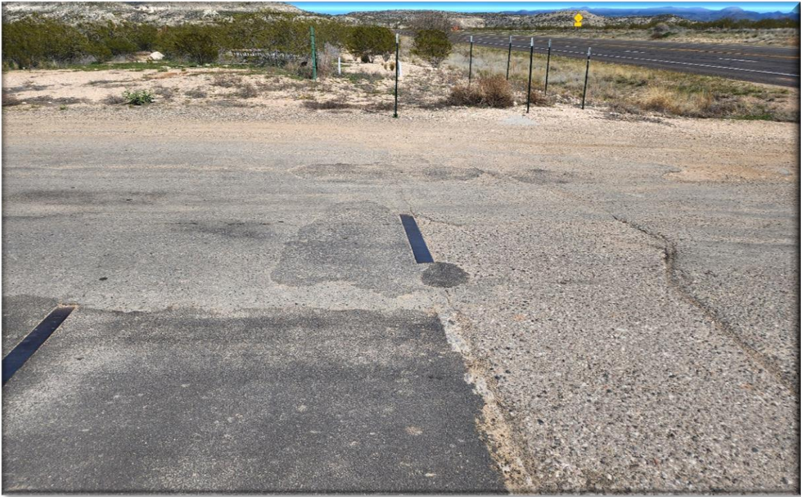
There is a foundation for an old cattle guard that needs to be removed at Highway 260.
