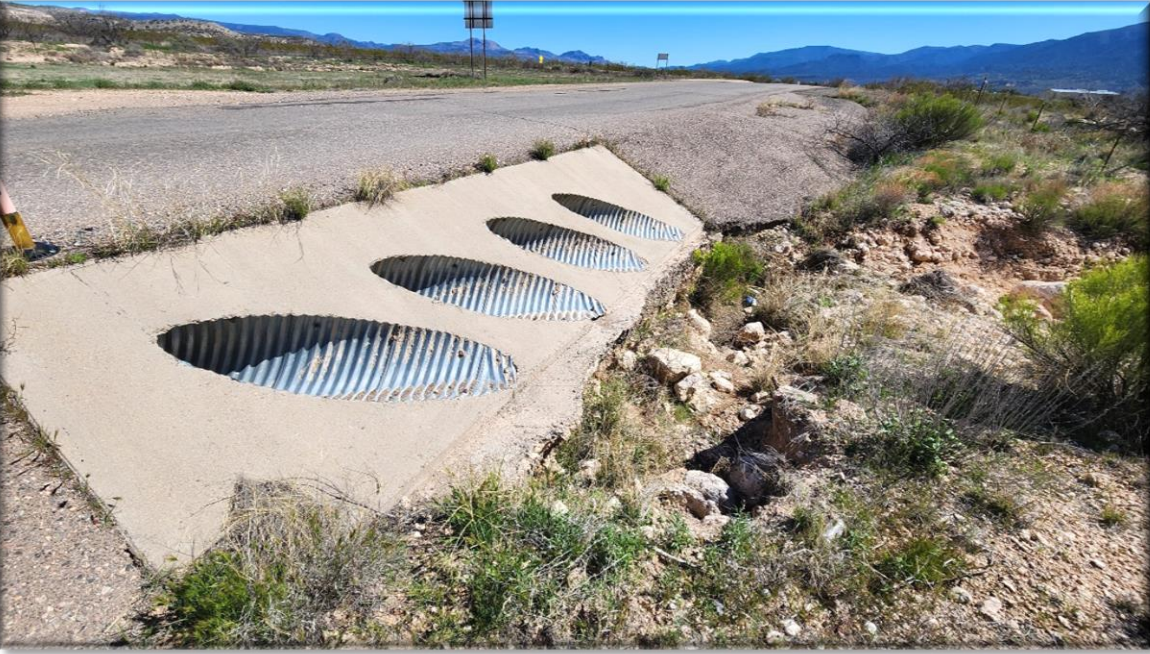
Erosion along the west side of Champion Trail needs to be repaired and stabilized.
