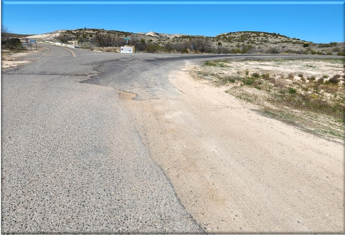
The intersection of Champion Trail and Cowboy Way. Note the repaired asphalt. This is due to the flow of stormwater across the intersection eroding the asphalt. Also note that the existing asphalt is only slightly wider than the southbound lane. Most of the northbound lane into the sports complex is dirt/rock.
