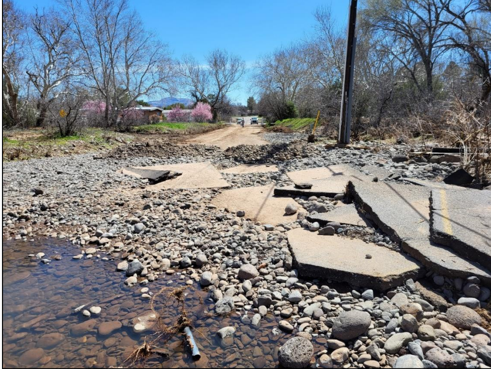
Photograph 2-5. Flooding aftermath at Verde Lakes Drive showing riverbed deposits and severe roadway damage.
