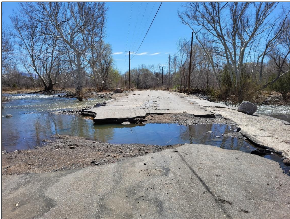
Photograph 2-4. Roadway damage at Verde Lakes Drive due to the March 2023 flooding event.
